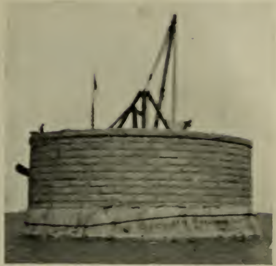
Wilson Avenue Crib, showing Masonry on Steel Shell. NEW WATER TUNNEL AT CHICAGO.
